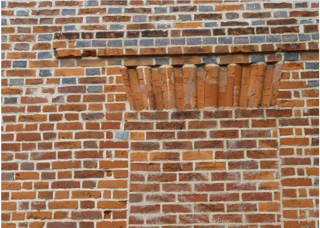
Contrast of brick coursing/poor mortar repairs
