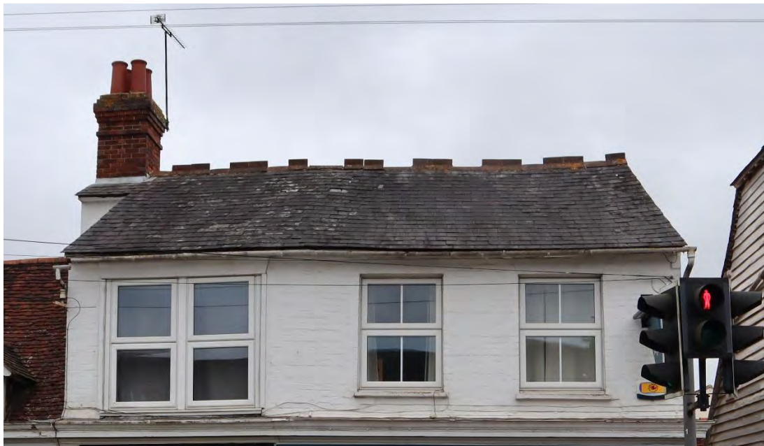
Figure 45 - UPVc double glazed windows change the character of the building, and cause harm to the Conservation Area.
